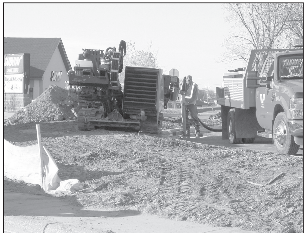
Construction workers at the site of the new McDonald's, working to get it up and running before winter.
